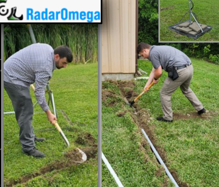
Pictured: Jordan Snyder, Infrastructure systems Supervisor (above), and Charles Zugaro, Infrastructure Systems Analyst (right) installing the cabling for the weather Station at Snider Tower.
